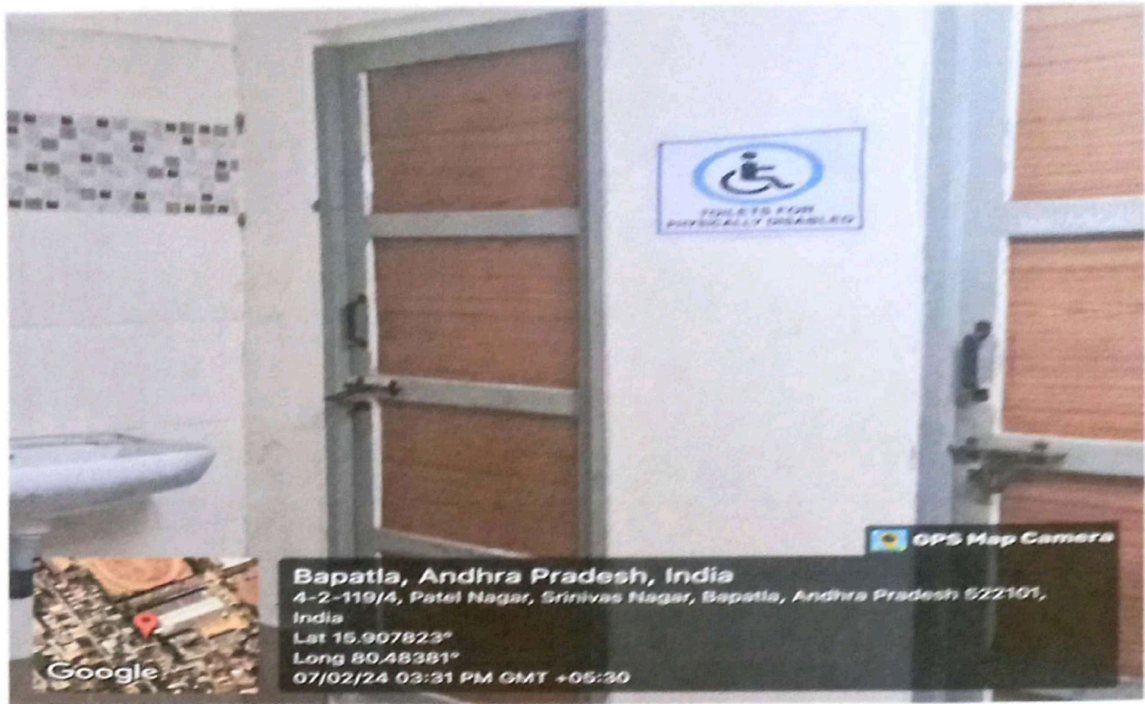
TOILETS FOR DISABLED PERSONS
